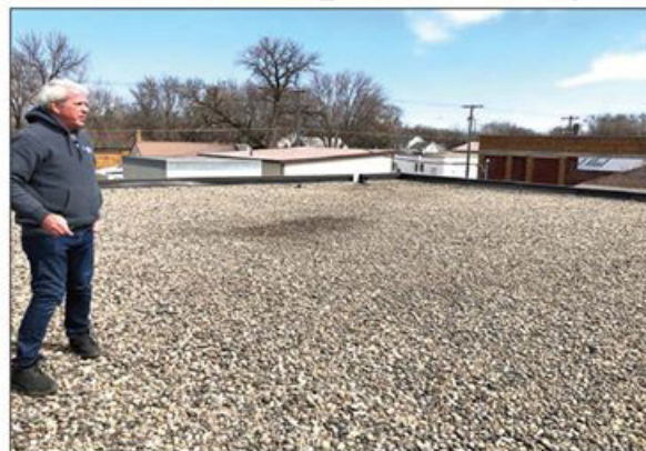
Before any work was done, Dave Laursen of MNSolar inspected the rooftop of the Kerkhoven Banner office to see what size solar array would work. Installation of the 56 solar panels was completed the last week of the year, and will be generating electricity for the building as soon as Otter Tail Power hooks them into the grid.
